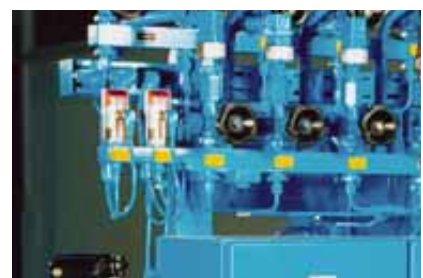
Essential: Temperature monitoring in air conditioning.
